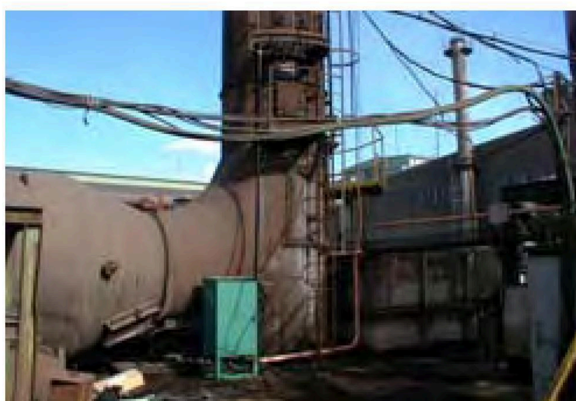
Chimney Bag Filter Exit
